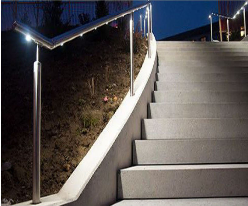
A. Railing Lights
