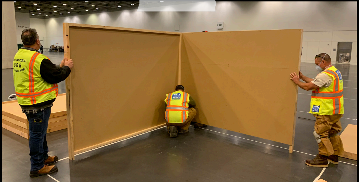
OUR CARPENTERS BUILD A POPUP SHELTER AT MOSCONE CENTER THAT PROVIDES PEOPLE WITH SEPARATED SLEEPING PODS FOR SAFE SOCIAL DISTANCING.
