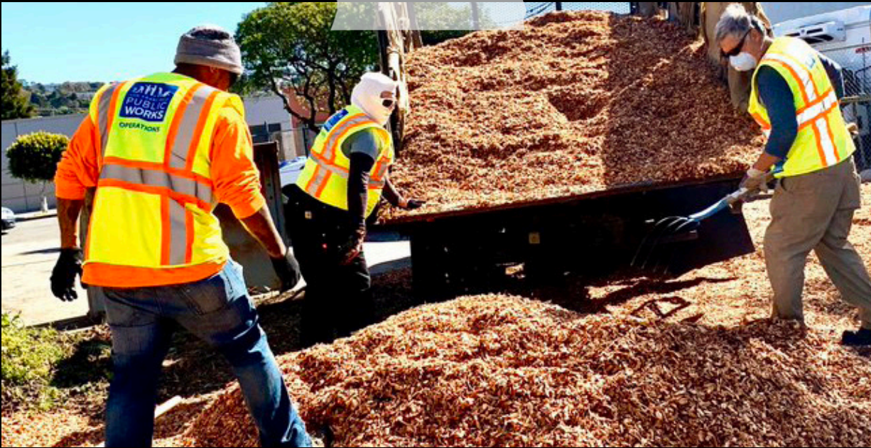
ALAN PAYNE WORKS THE BACKHOE TO GRADE A LOT, AS HE AND OTHER MEMBERS FROM OUR STREET REPAIR AND LANDSCAPING CREWS PREPARE A NEW COVID-19 TESTING SITE IN THE SOMA NEIGHBORHOOD.
