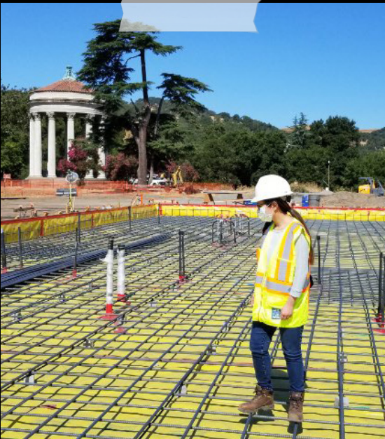
TINA KWAN WITH OUR STRUCTURAL ENGINEERING TEAM IN SUNOL, WORKS ON THE ALAMEDA CREEK WATERSHED CENTER.
