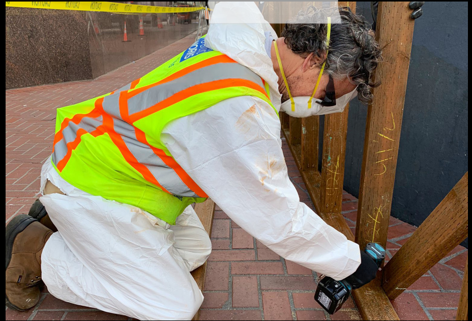
OUR CARPENTERS CONSTRUCT STURDY SAFETY BARRICADES TO CLOSE OFF THE MUNI STATION ENTRANCES ON MARKET STREET.
