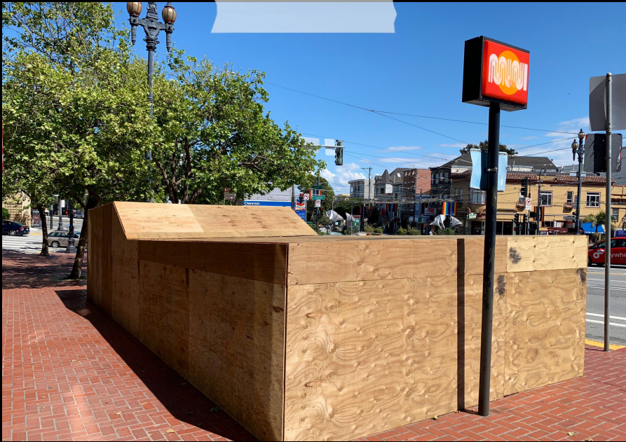
WHEN MUNI SUBWAY SERVICE SHUT DOWN FOR THE COVID-19 PUBLIC HEALTH EMERGENCY, OUR CARPENTERS ANSWER THE CALL AND SECURE THE METRO STATIONS.
