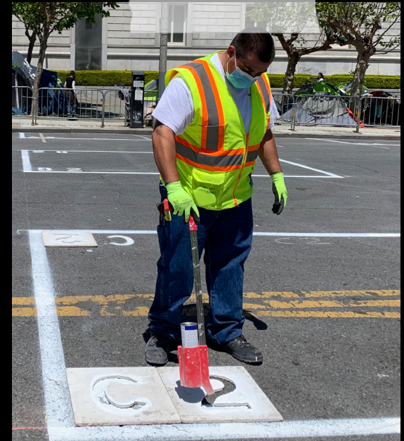
OUR PAINTERS PREPARE THE SAFE SLEEPING SITE ON FULTON STREET, CREATING SOCIALLY DISTANCED TENT SPACES.
