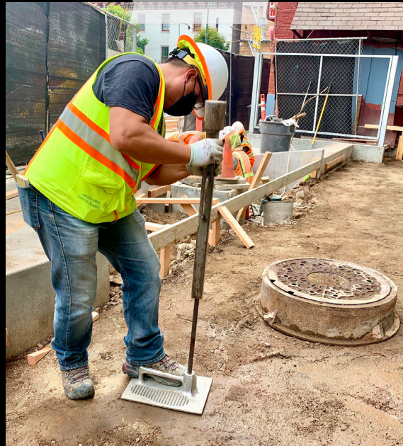
SOIL COMPACTION GETS TESTED DURING THE RENOVATION OF THE WILLIE "WOO WOO" WONG PLAYGROUND IN CHINATOWN.
