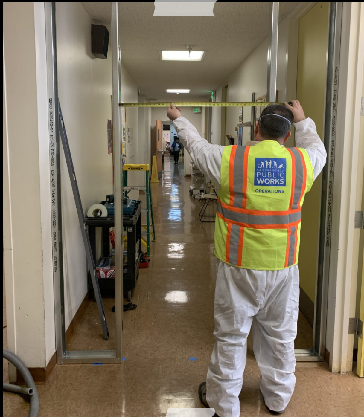
DAVID HERNANDEZ, CARPENTER, WORKS ON A COVID-19 SAFETY PROJECT AT A NEIGHBORHOOD HEALTH CENTER.
