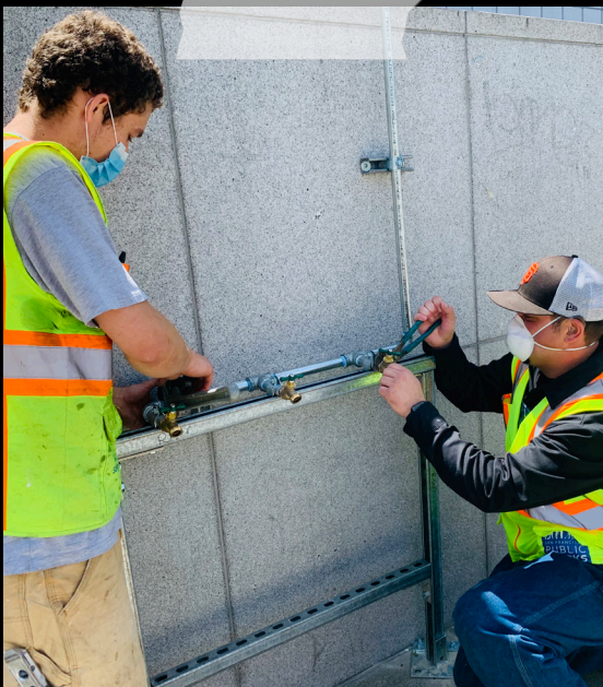
OUR PLUMBERS SET UP ACCESS TO FRESH WATER AT THE FULTON STREET SAFE SLEEPING SITE.
