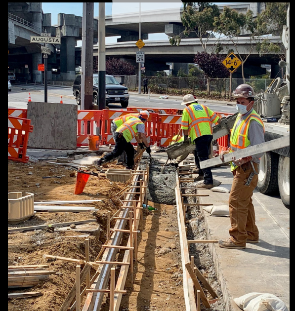
CEMENT SHOP CREWS POUR A NEW SIDEWALK AND ADA-COMPLIANT CURB RAMPS IN THE SILVER TERRACE NEIGHBORHOOD.
